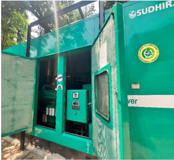
Figure 7 New generator set with 1000 KW capacity
