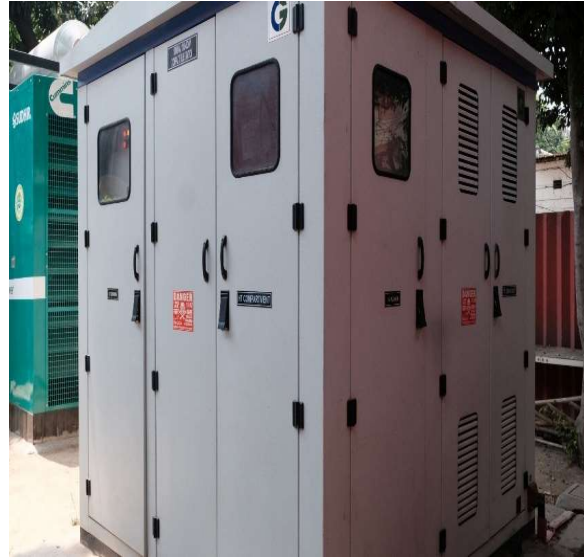
Figure 8 New transformer of 500 KVA capacity
